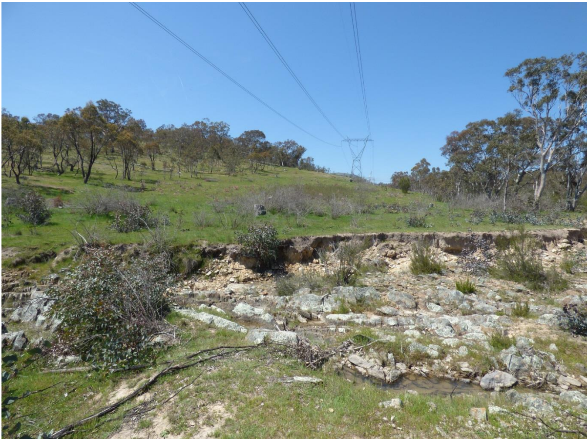
Figure 19 Erosion occurring as a result of surface runoff from upslope area
