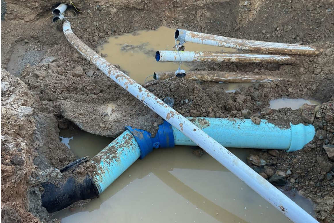
Figure 1.3.5 Service crossing resulting in damaged thrust block
