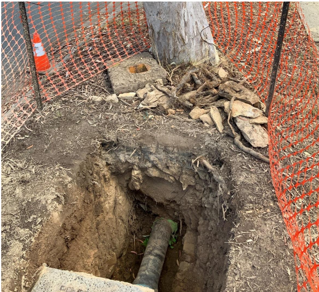
Figure 1.3.4 Tree roots impeding access to water main
