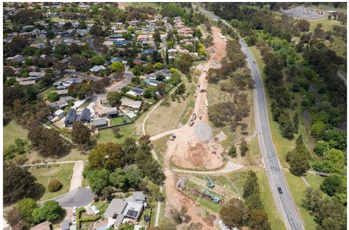
A bird's eye view of the new sewer trunk main being installed adjacent to Ginninderra Drive
